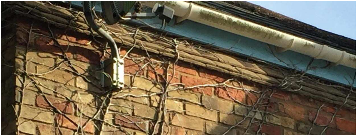
Detail of a portion of the earlier roof now covered by secondary roof structure and slate tiles, probably added as part of the 1956 remodelling of the building.
